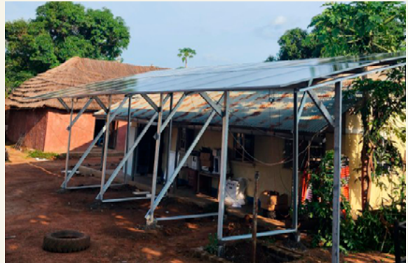
Solar PV and Battery System at our Mundri Field Office, South Sudan.
